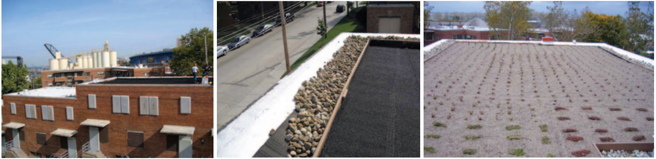
GROWING TREND Using materials manufactured, propagated and installed by local companies, vegetative roofs were recently installed on seven of 13 Cleveland Metropolitan Housing Authority buildings as part of a system-wide renovation project.
